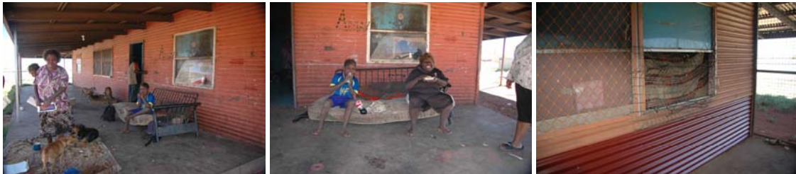
Michael Bulla and Nellie Mick's house # 35 – leaks fill the kitchen with water and windows and doors are not secure
