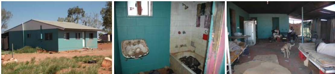
Pauline Smith's house # 57 – outside was painted but the house is still uninhabitable
