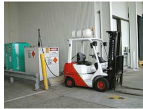
Forklift CNG station
