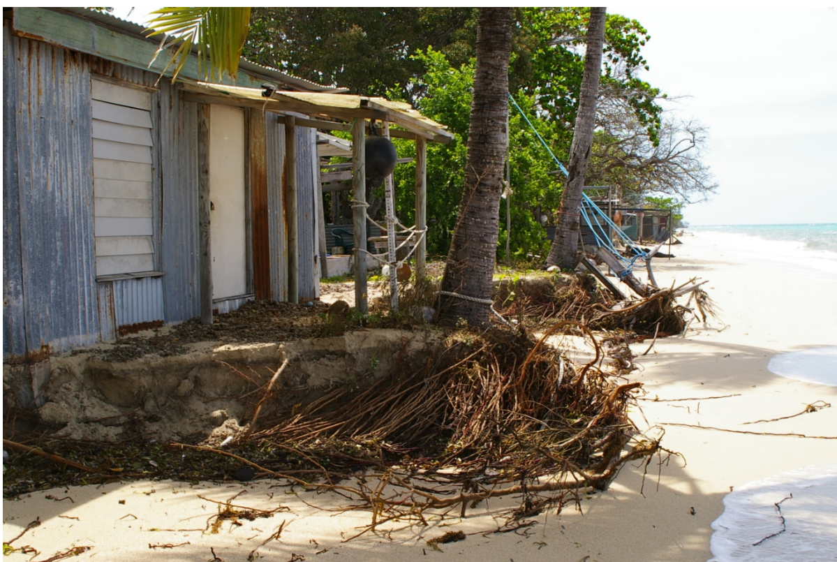
Shoreline erosion on low lying islands in the Torres Strait
