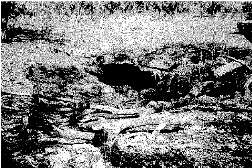
Plate 9 Example of a sinkhole formed by cave roof collapse, located north of Zimin Drive and east of Florina Road
