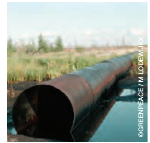
image Oil spill and pipelines in Nizhnevartovsk, West-Siberia
