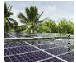
image SOLAR PANELS ON REFRIGERATION PLANT (FOR KEEPING FISH FRESH). LIKIEP ATOLL, MARSHALL ISLANDS.
