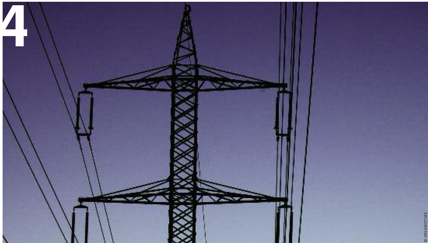
image ELECTRICITY LINES.
