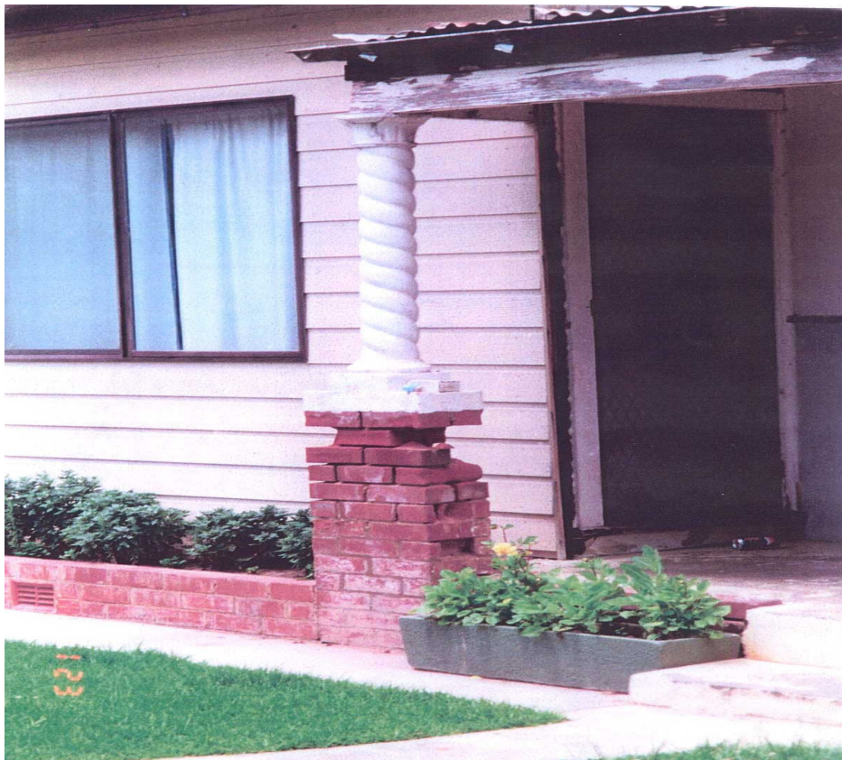
Photograph: Salinity damage to brickwork, Wagga Wagga, NSW
