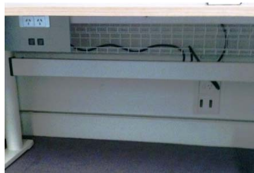
Neat arrangement of cables in tray
