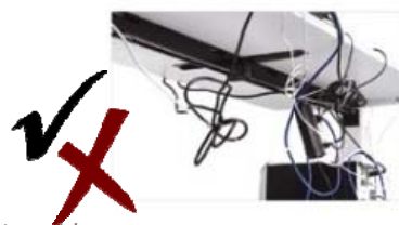
No cable management system = messy cables
