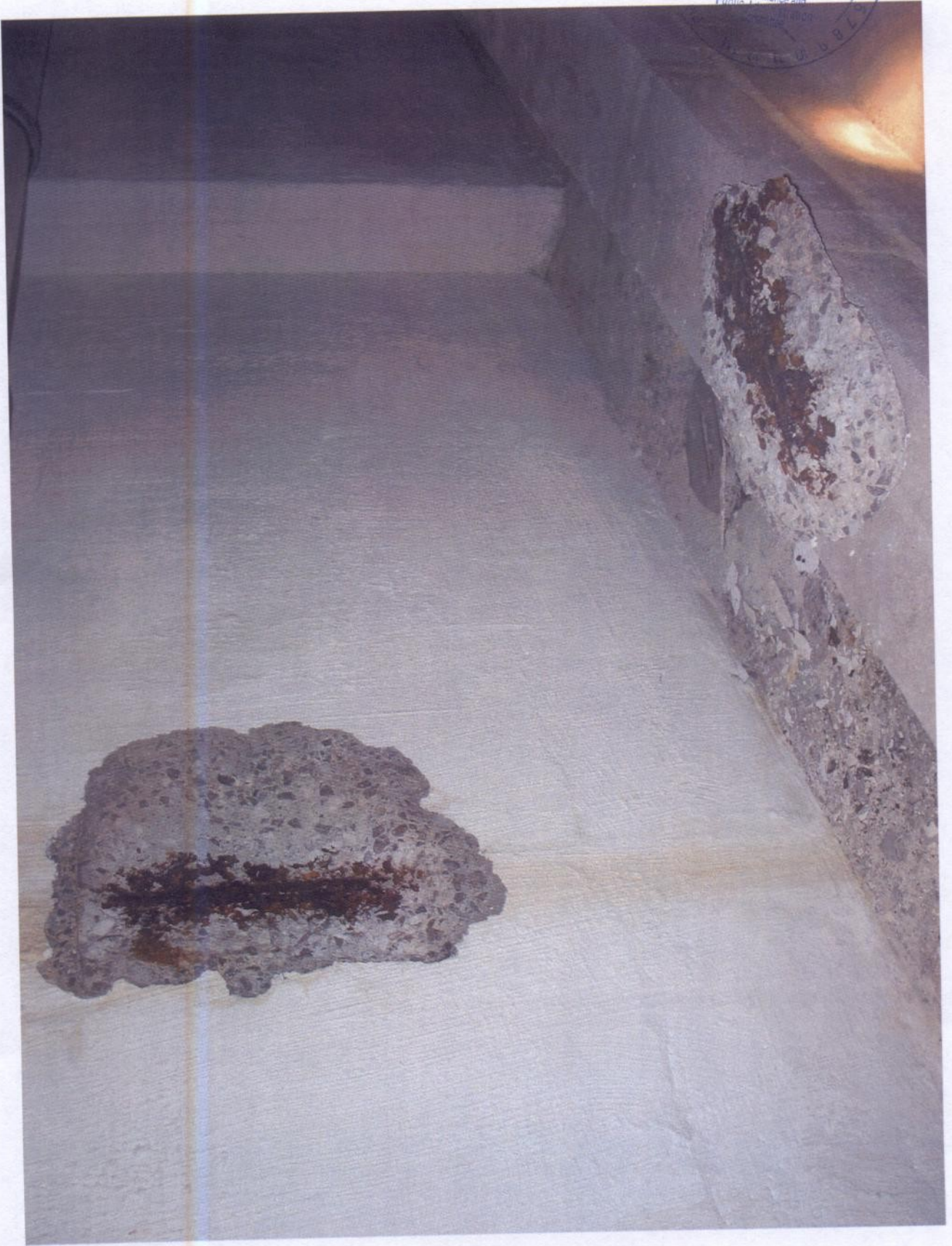
Attachment 1 – Corrosion of reinforcement resulting in concrete spalling (Eastern wall)
