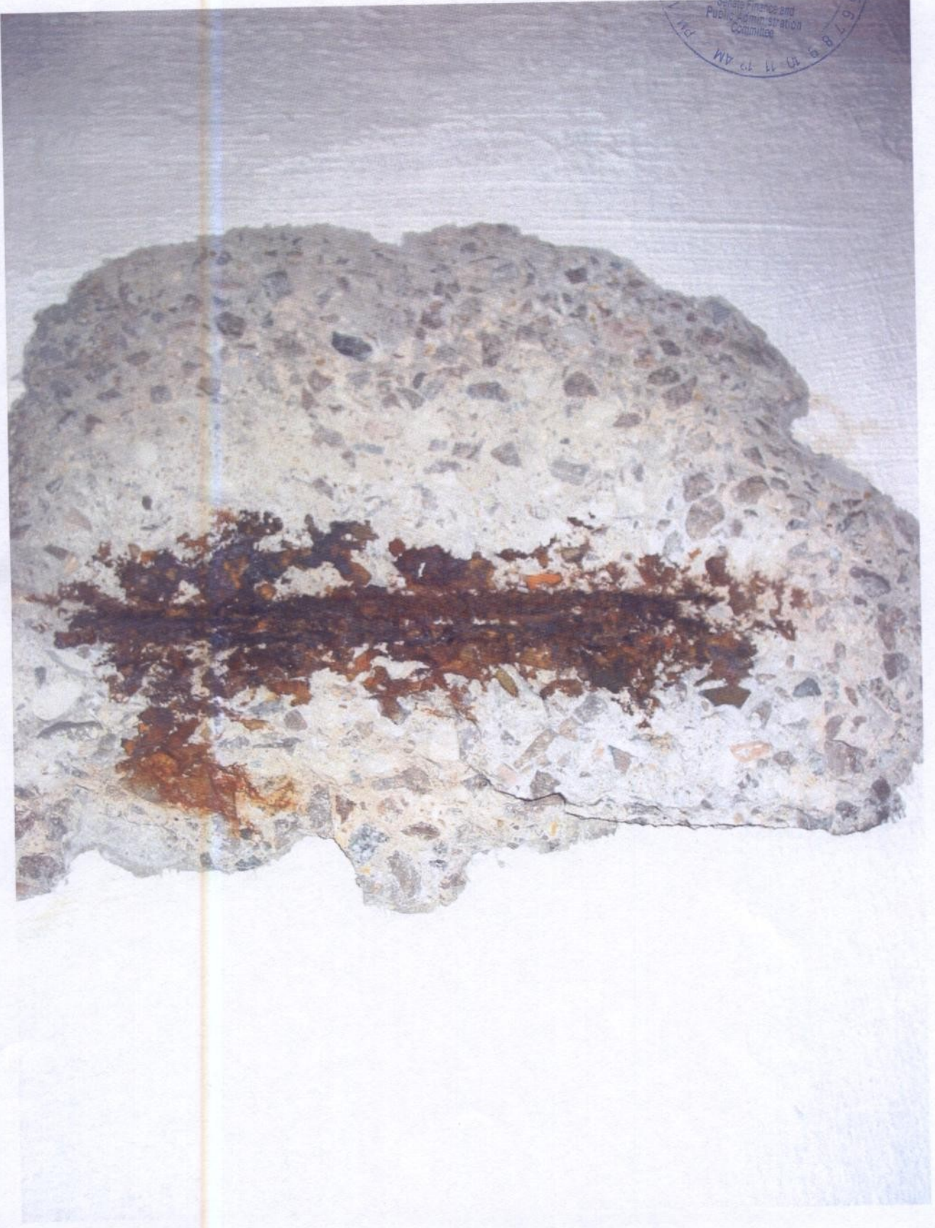
Attachment 2 – Close-up of reinforcement corrosion (Eastern wall)
