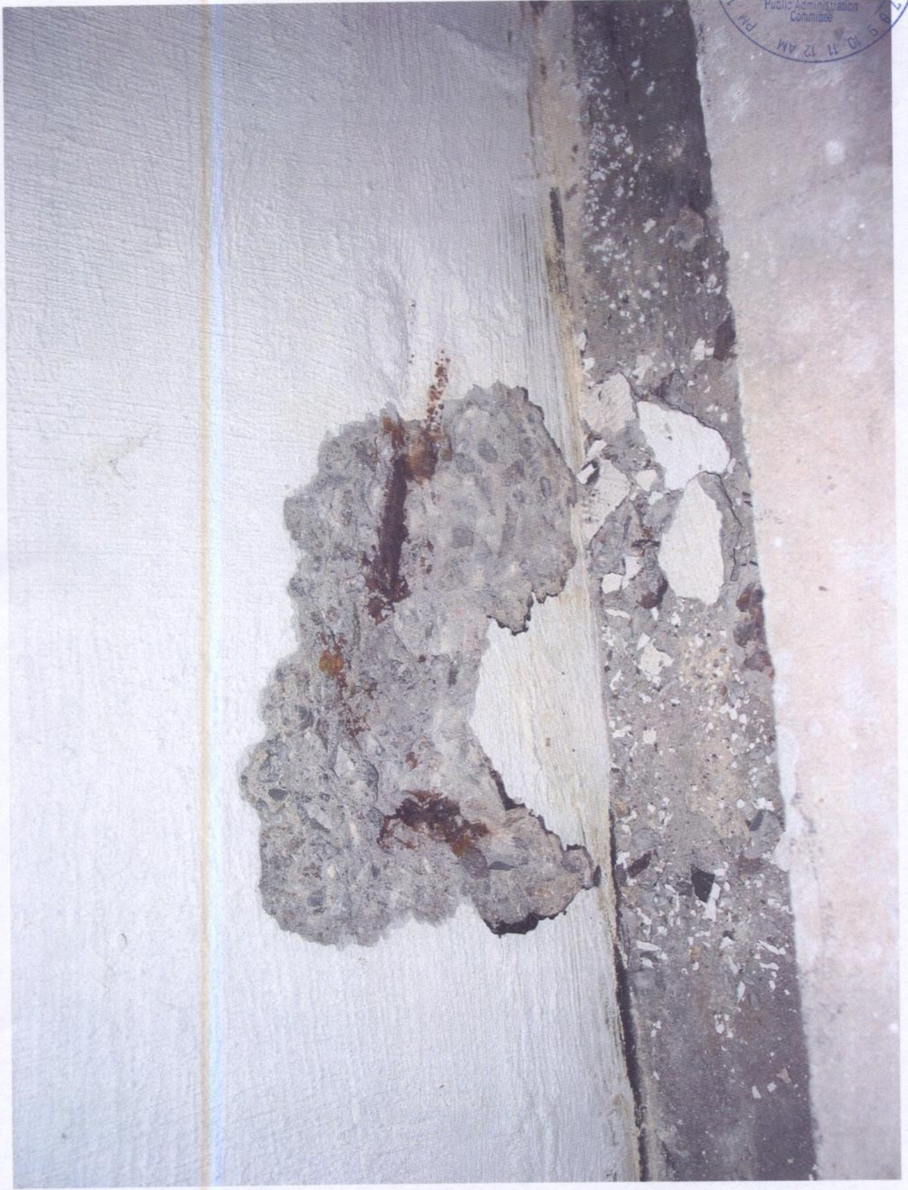
Attachment 3 – Corrosion of reinforcement resulting in concrete spalling (South wall)
