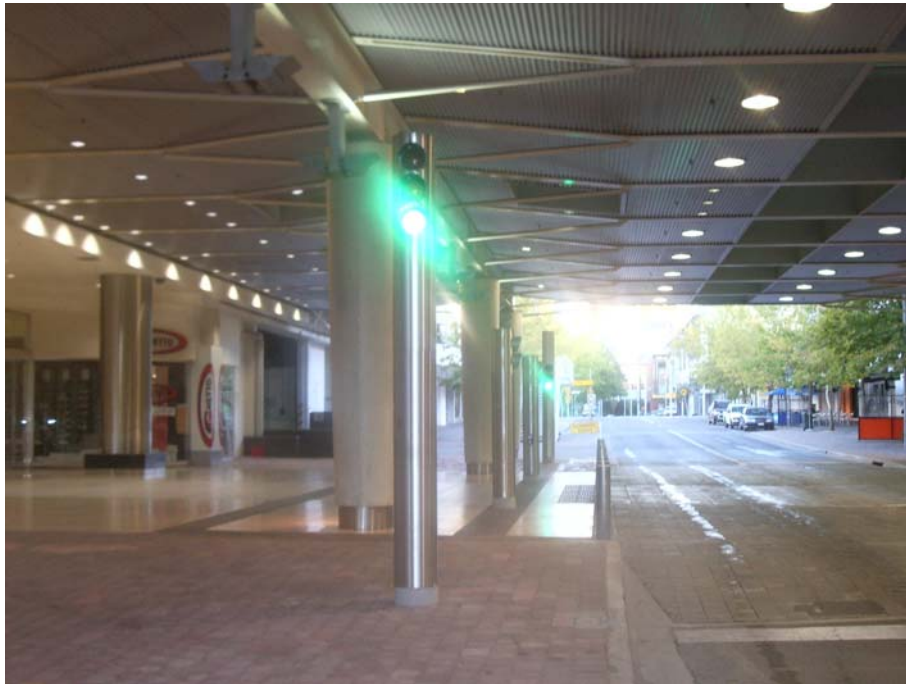
Stainless Steel traffic signal hardware used on Bunda Street at the Canberra Centre.
