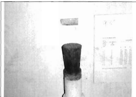
6-133-1-W sounding pipe plugged
