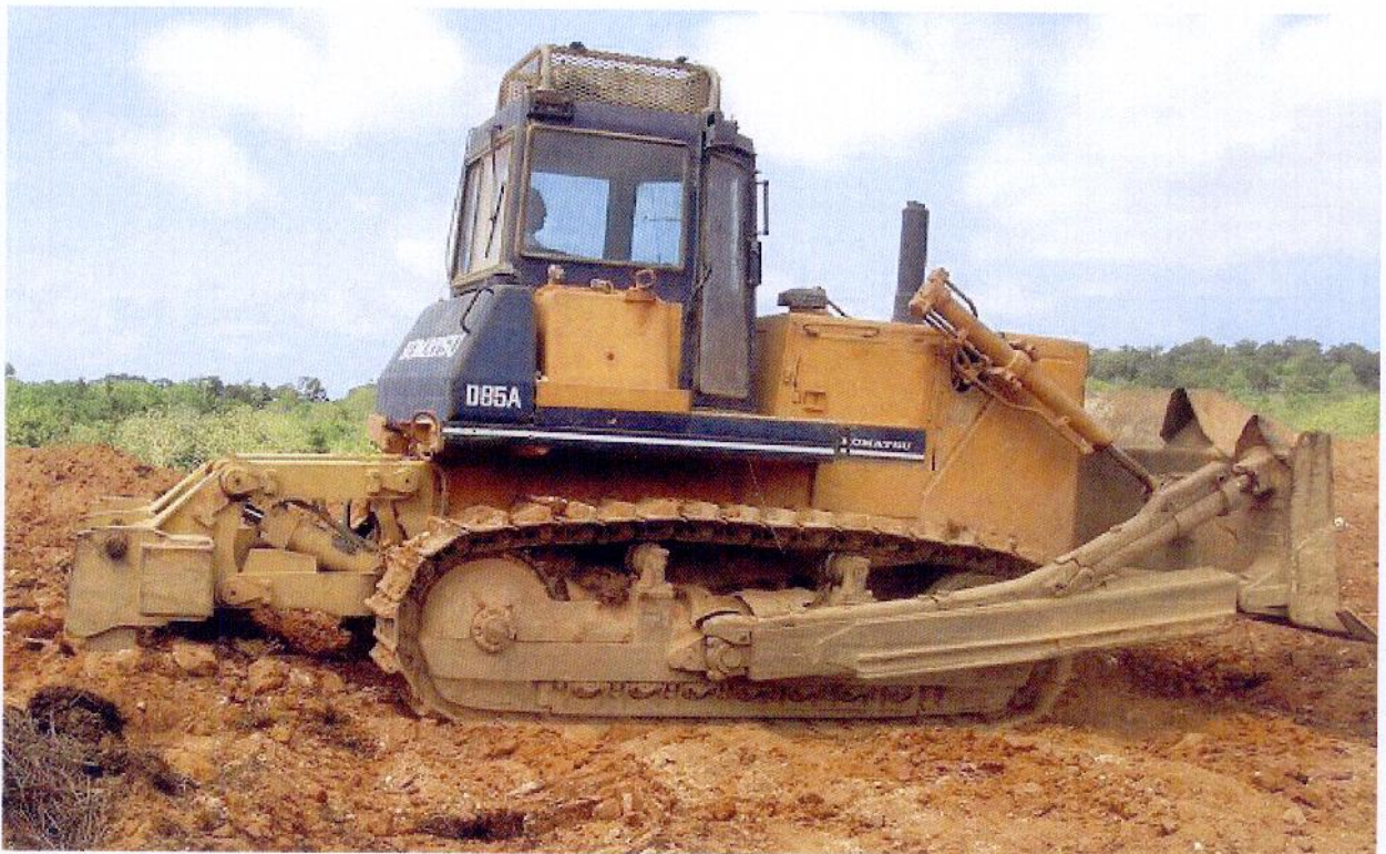
Figure 8: D8 dozer doing a final rip of planting beds in mine field 20C before planting.
