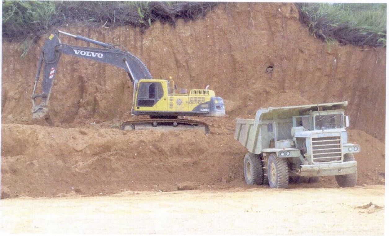
Figure 7: Earthmoving contractors loading 30 tonne dump trucks from a stockpile at mine field 20C.
