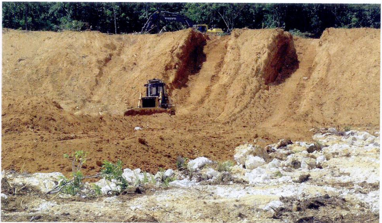
Figure 6: Earthmoving contractors slotting stockpiles to build up the soil profile in the adjacent abandoned section of mine field 20E.
