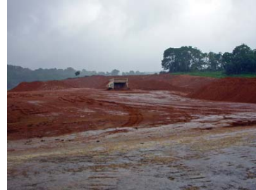
Figure 11: IRPC construction site on 13 October 2006, showing remnant, secondary regrowth in the foreground
