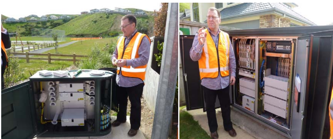
NZ Figure 5 A Chorus representative showing the cabinet infrastructure supporting the copper and fibre networks
