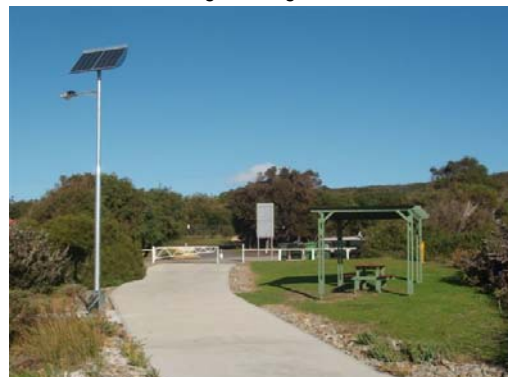
Solar-powered light over fish cleaning table and pergola
