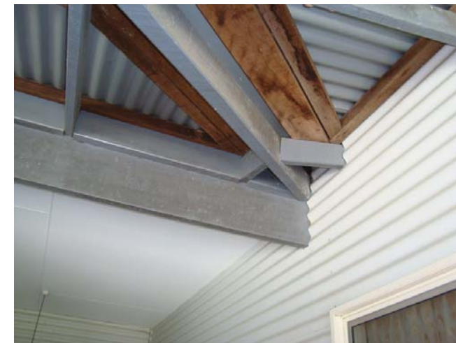
Where roof pitch changes at valley, roof leaking and damaging floor below. Leaking exacerbated by low pitch to verandah
