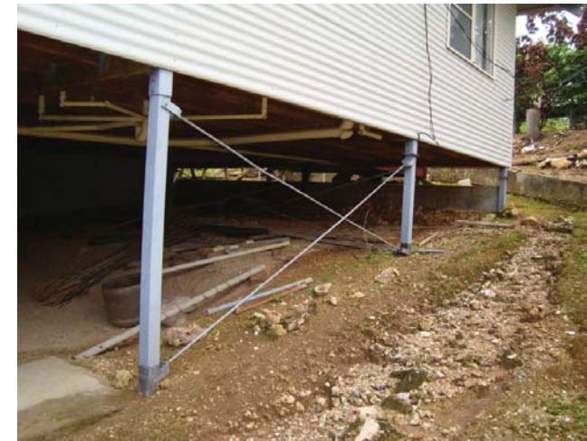
Unscreened sub-floor unattractive and area dangerous for children as it is accessible. Needs to be screened, with lockable access door
