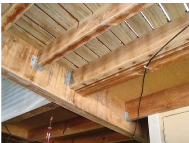
Stained pine decking, rotting where exposed to elements on upper floor. Main flooring rotting, inappropriate material.
