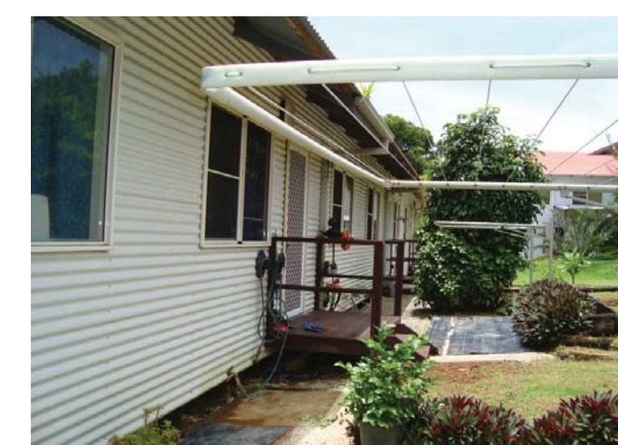
Screws not appropriate to marine environment - rusting. Where water drips on timber, timber is rotting.
