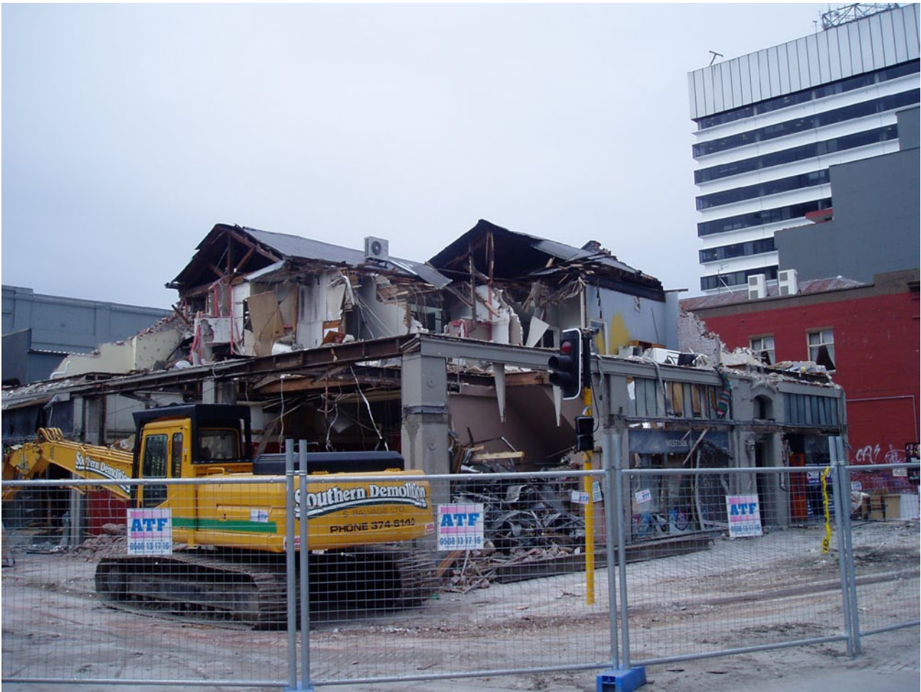
Photo: Christchurch Earthquake damage.
