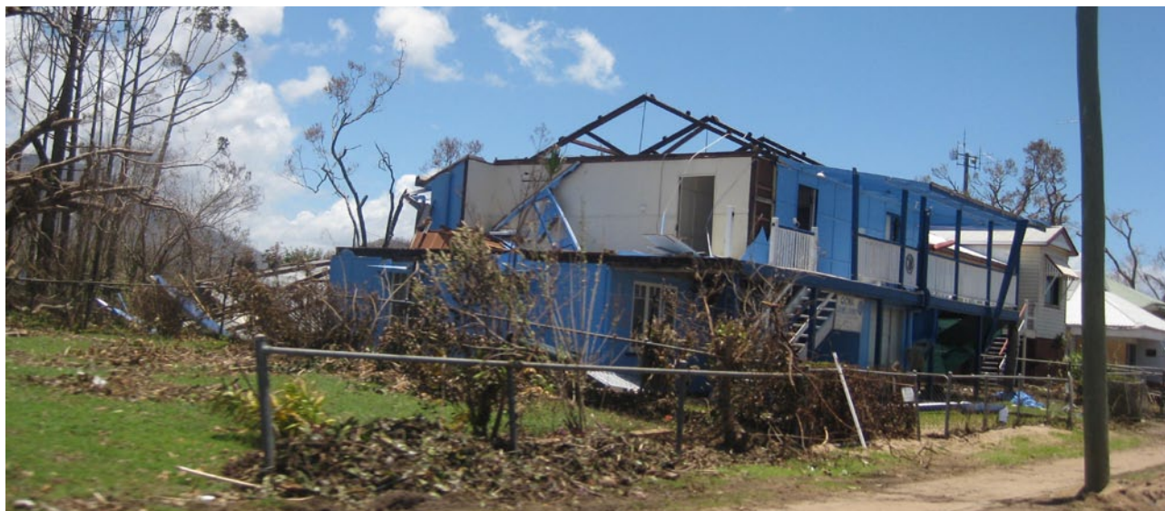
Photo: Cyclone Yasi damage, 2011.
