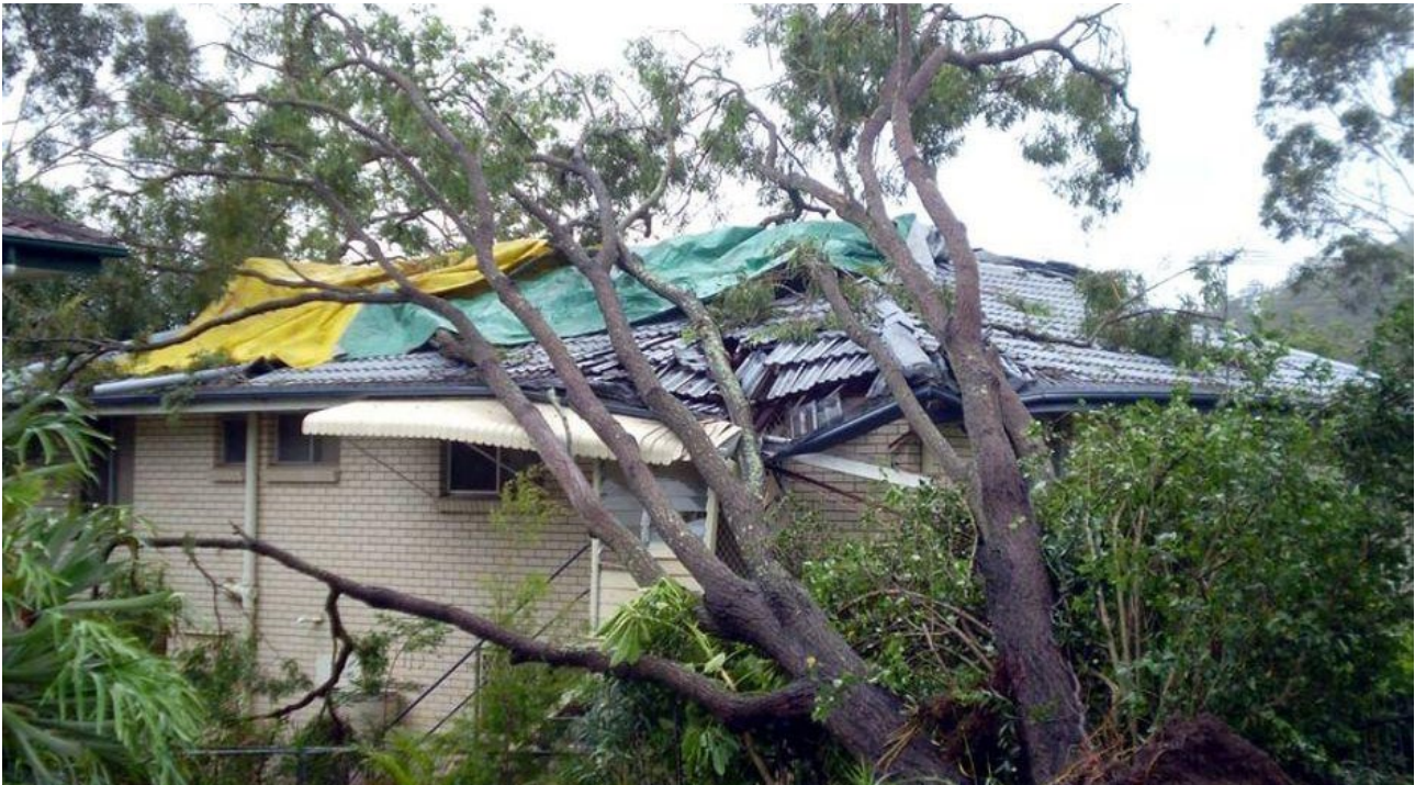
Photo: Severe storms cause roof damage in The Gap, Brisbane on 16 November 2008.
