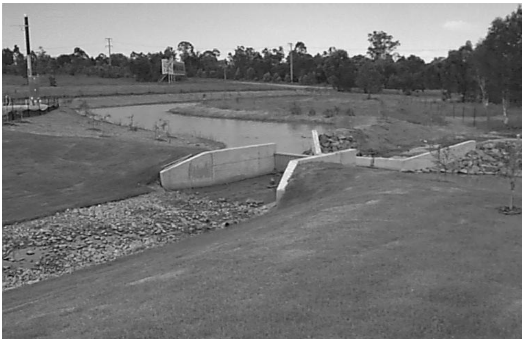
Plate 1– Catchment Management Infrastructure (iTrash Rake, Silt Trap & Artificial Wetland)
