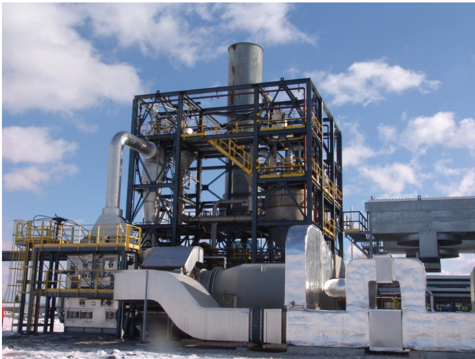
200 tonne per day wood pyrolysis plant at Guelph in Ontario, Canada. Similar plants are proposed for Western Australia.
