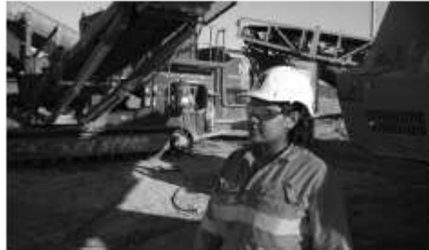
Narassa, Northern Project Contracting, on site at Century Mine in the Gulf of Queensland
