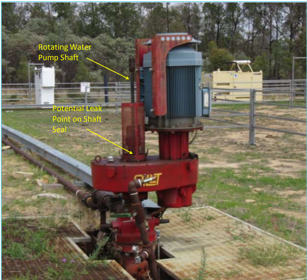
Figure 5.3. Well head showing the location of the water pump shaft and seal which was found to be a common leak point.
