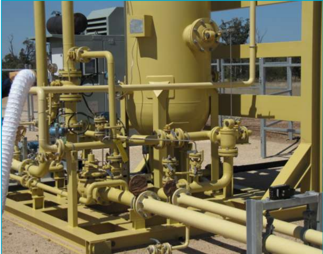
Figure 4.3. CSG well pad showing some of the surface equipment and potential emission points. Note the engine in the background for supplying hydraulic power to the water pump.
