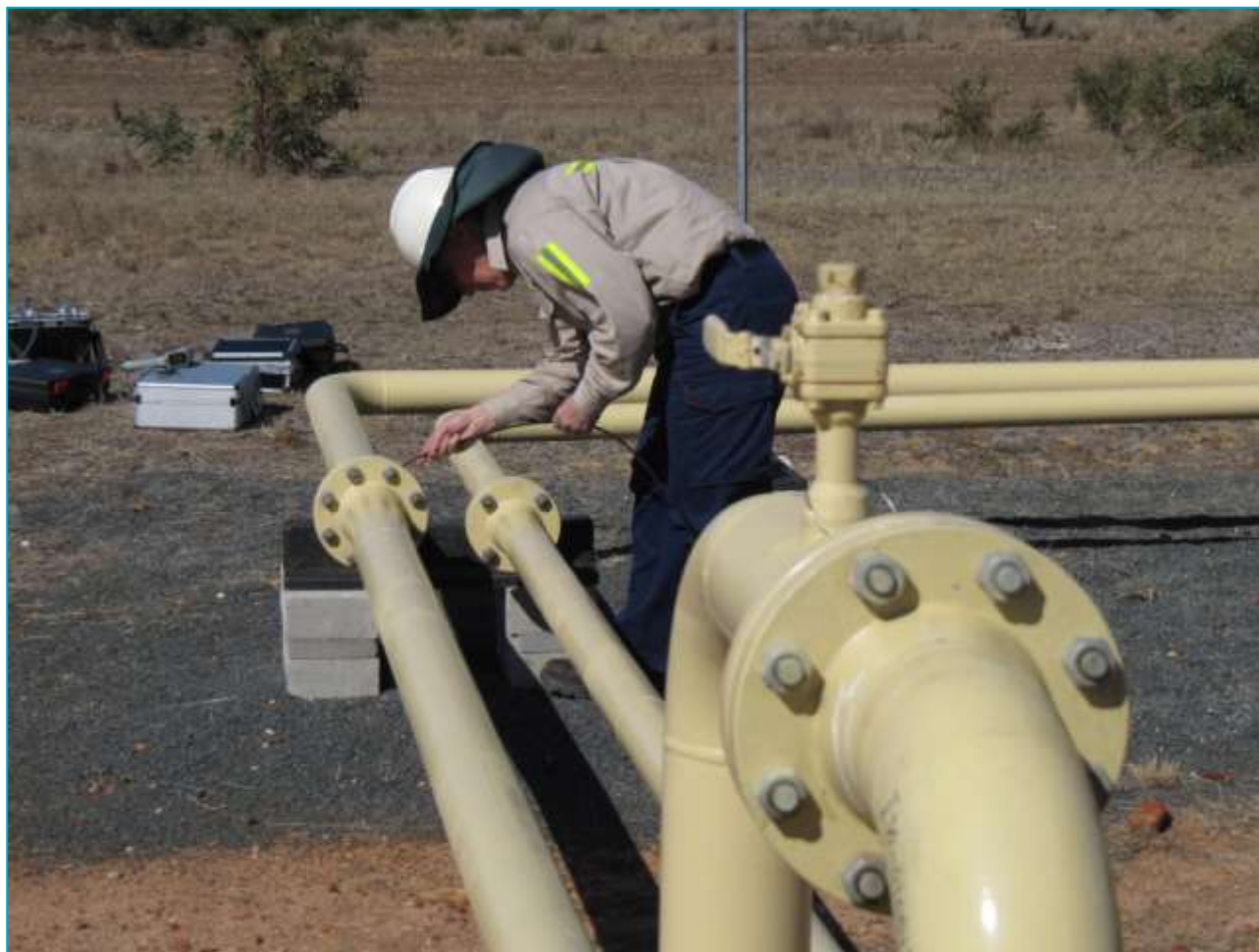
Figure 3.4. Locating equipment leaks at a CSG well pad.
