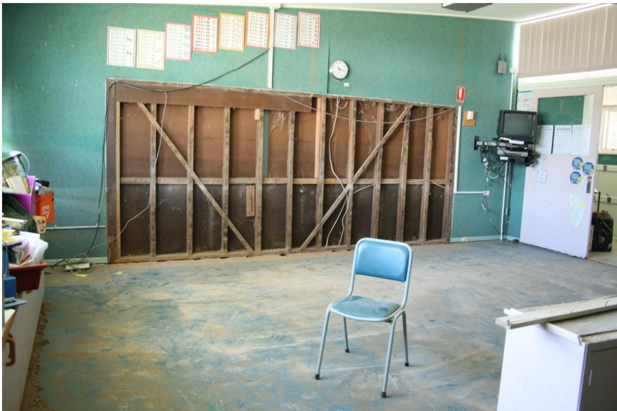
The front wall of the Senior Classroom where black boards have been removed to allow new joinery, whiteboards and existing electronic whiteboard to be installed.
