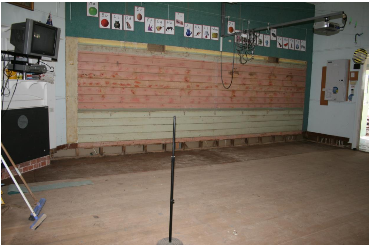
The front wall of the Junior classroom where blackboards, cupboards and a stage had been removed to allow new whiteboards and joinery and existing electronic whiteboard to be installed.
