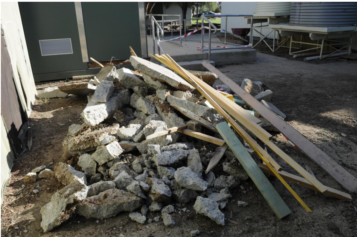
Rubble outside the main school building, which lay between the toilets and the playground for the entirety of Term 1.
