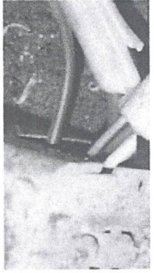
Damaged cable Sheaths
