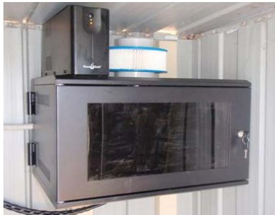
Radio Transmitter in 19” rack
