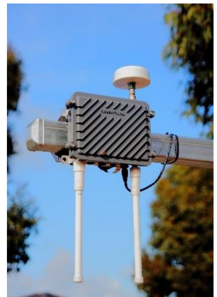
Figure 2: Roadside infrastructure for vehicle-to-infrastructure communications
