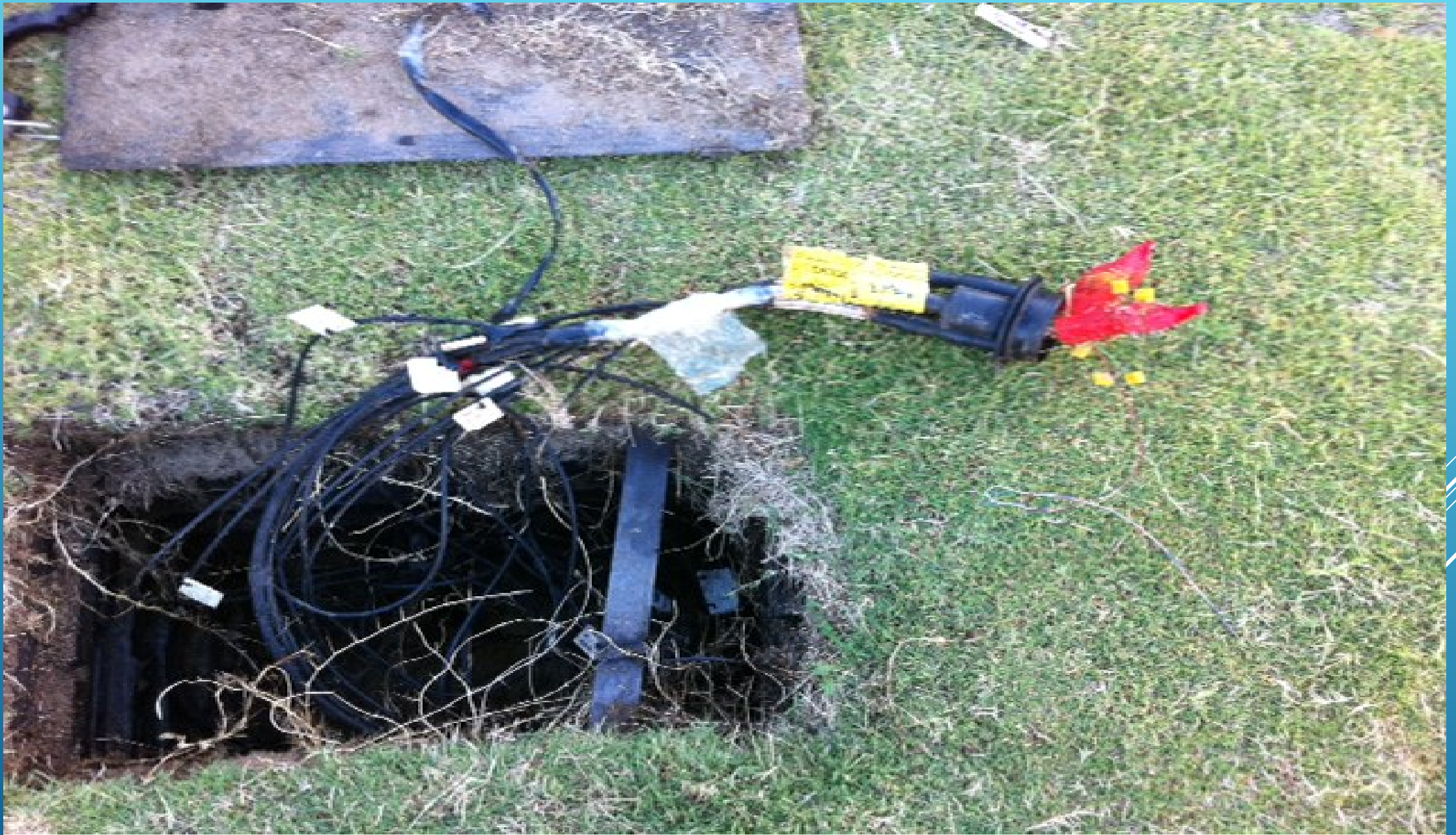
Photo: Energy in the network Project: Powerline GPS: 52.020000, 10.000000 Date: 2023-01-10 10:00:00
