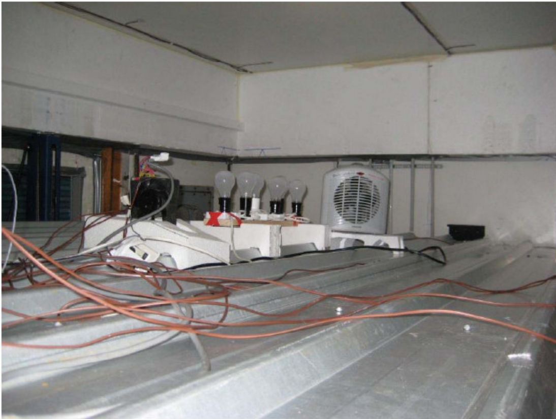
Figure 8. View from above roof, just after it has been lowered, showing heaters.
