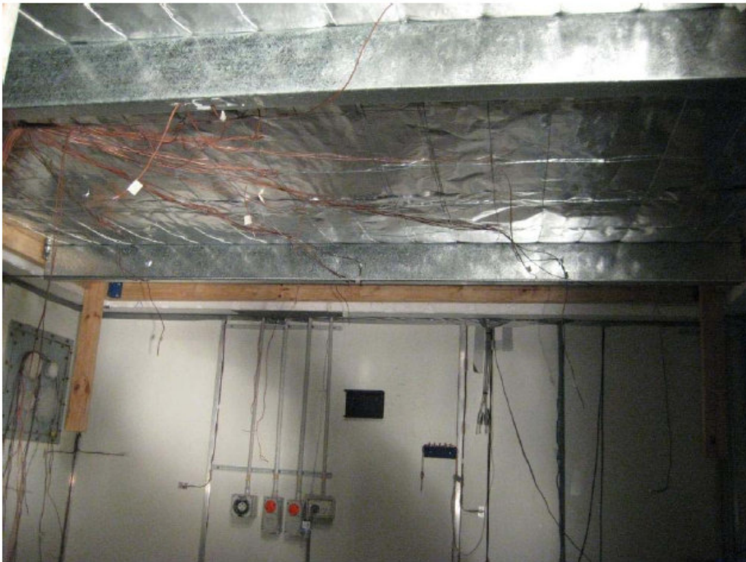
Figure 6. View from below of roof, as installed for test, showing blanket foil with thermocouples attached.
