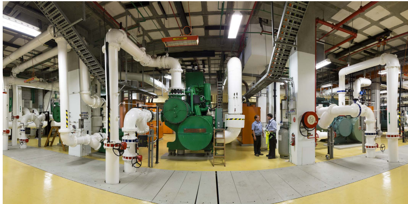
Maintenance Officer and Mechanical Fitter, Chillers Plant Room, 2014 Inkjet print 80cm x 160cm Parliament House Art Collection, Canberra
