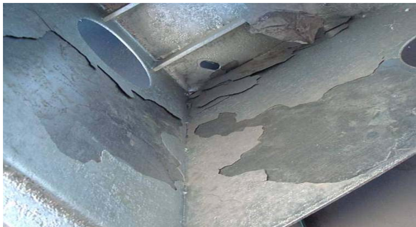
Photo 2 Poor galvanizing due to steel chemistry
