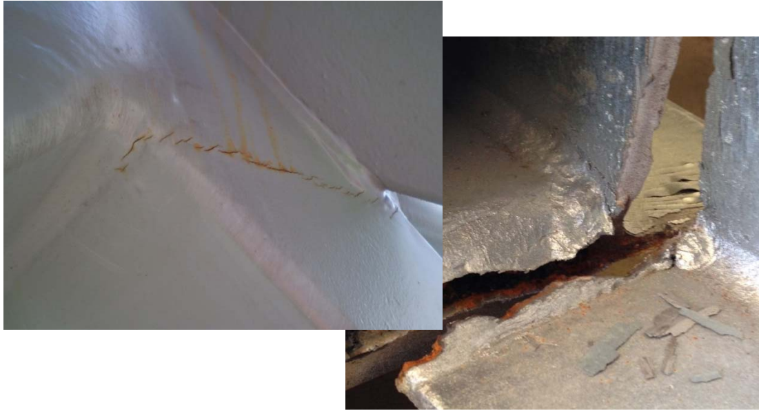
Photos 7–8 Steel cracking on imported fabricated product
