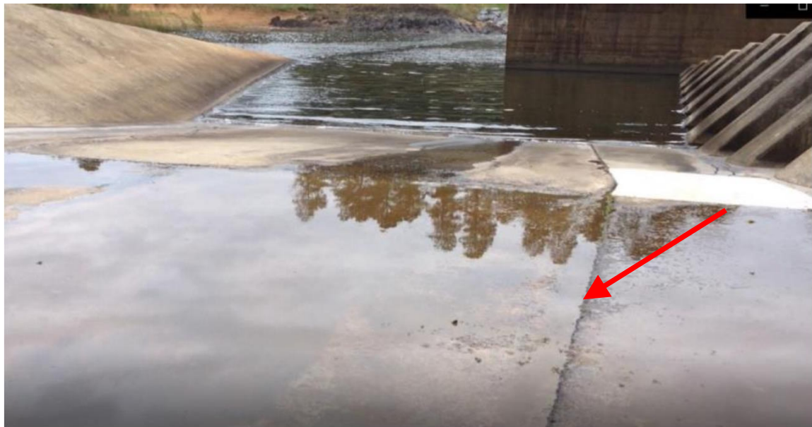
Figure 5: Bubbling between the Dissipator slab joints
