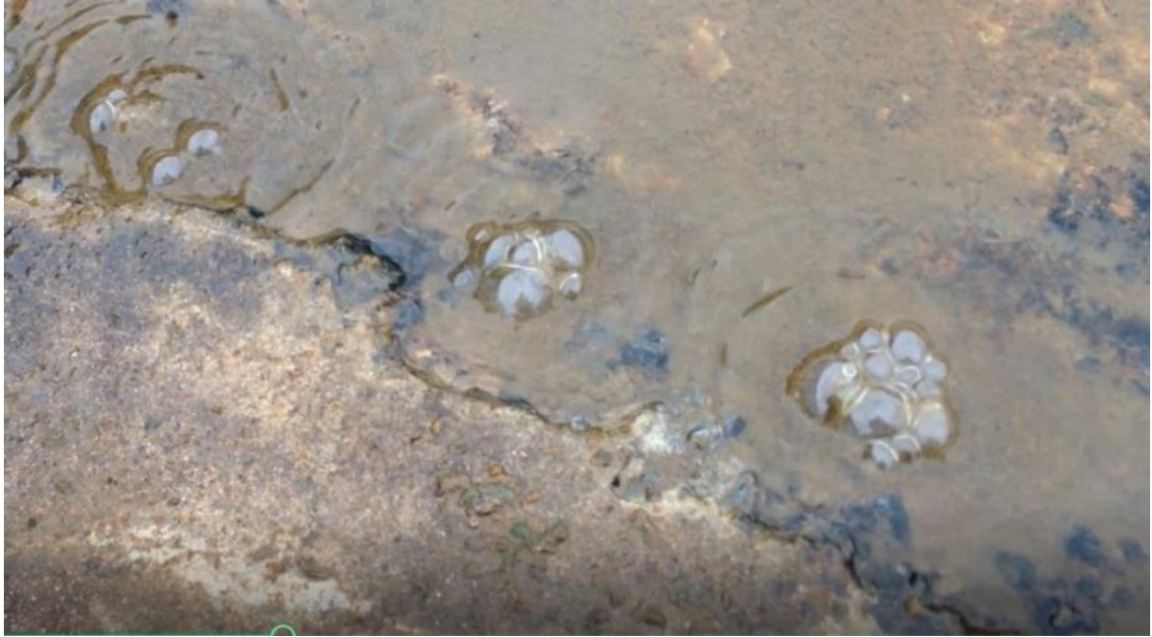
Figure 6: Close up bubbling between the dissipator slab joints
