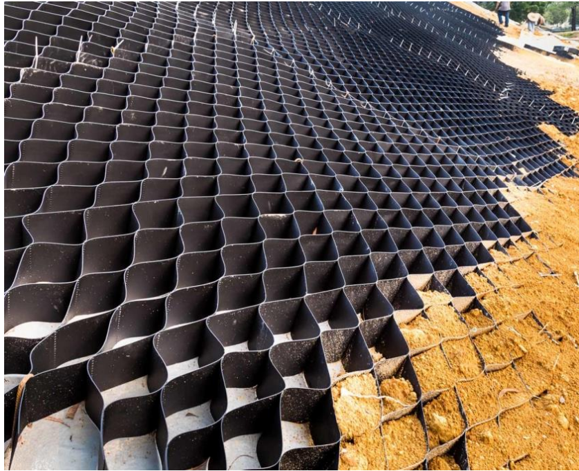
Figure 15: Indicative erosion protection matting to be placed on abutments and grassed over. (Image from Varsity Inc.)
