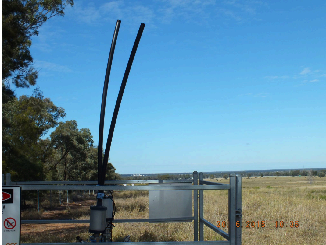
High point vent, photo courtesy of gas field visitor
