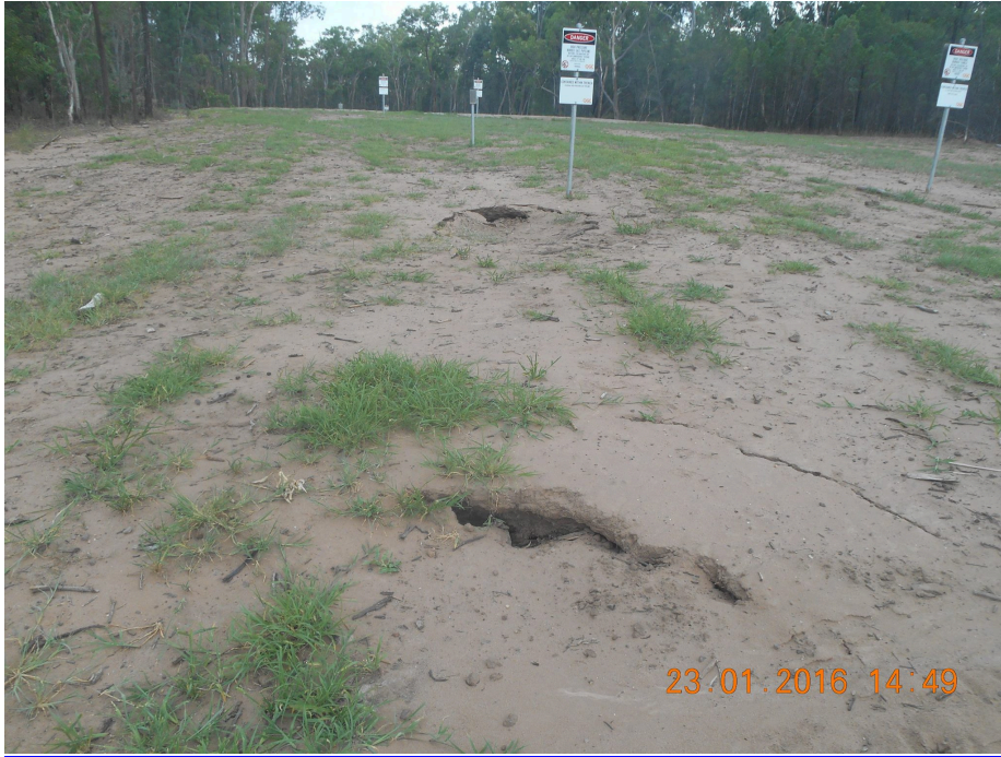
Subsidence along the gas pipeline photo courtesy of local resident
