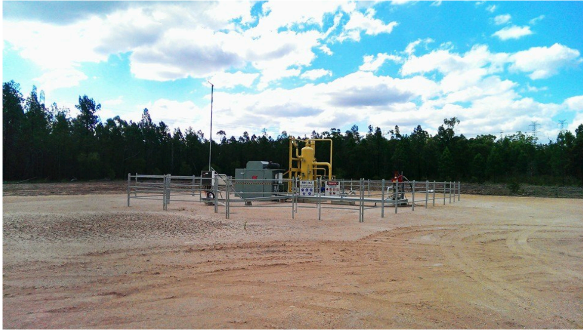
Gas infrastructure in state forest, photo courtesy of local resident
