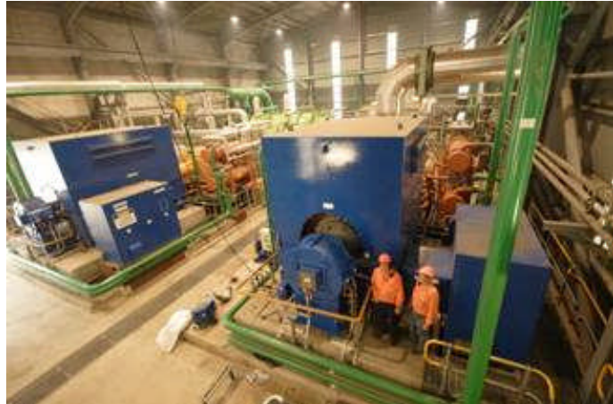
This is the turbine hall of CSR's $150 million Pioneer Sugar Mill cogeneration facility commissioned in 2006. The opportunity for more such facilities across the sugar industry could be lost if taxation-favoured forestry continues to intrude on commercial sugarcane farming operations.
