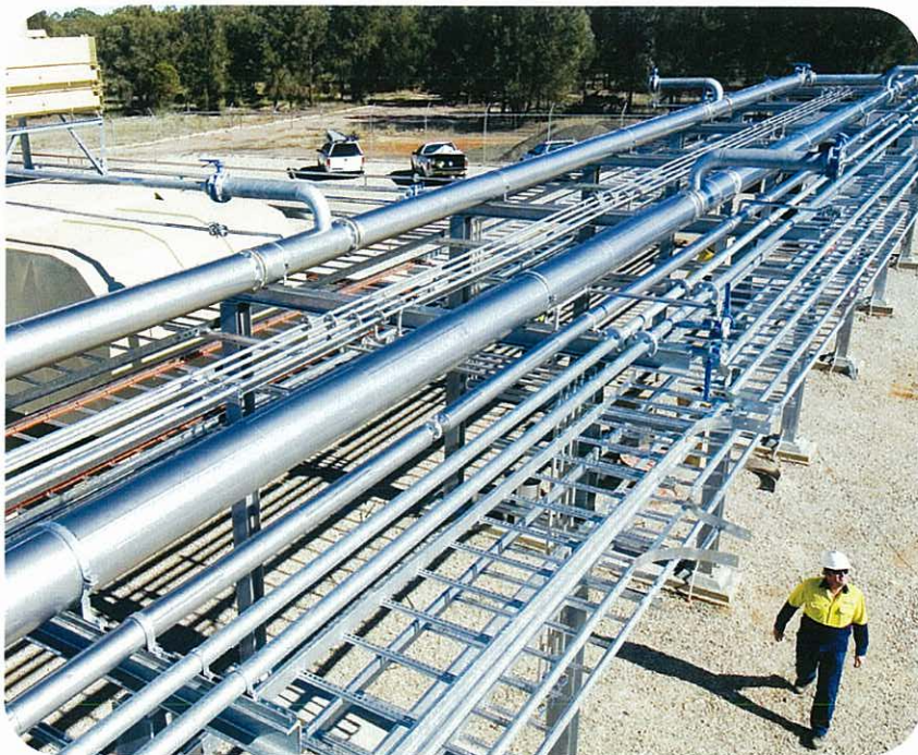
Wilga Park Power Station
