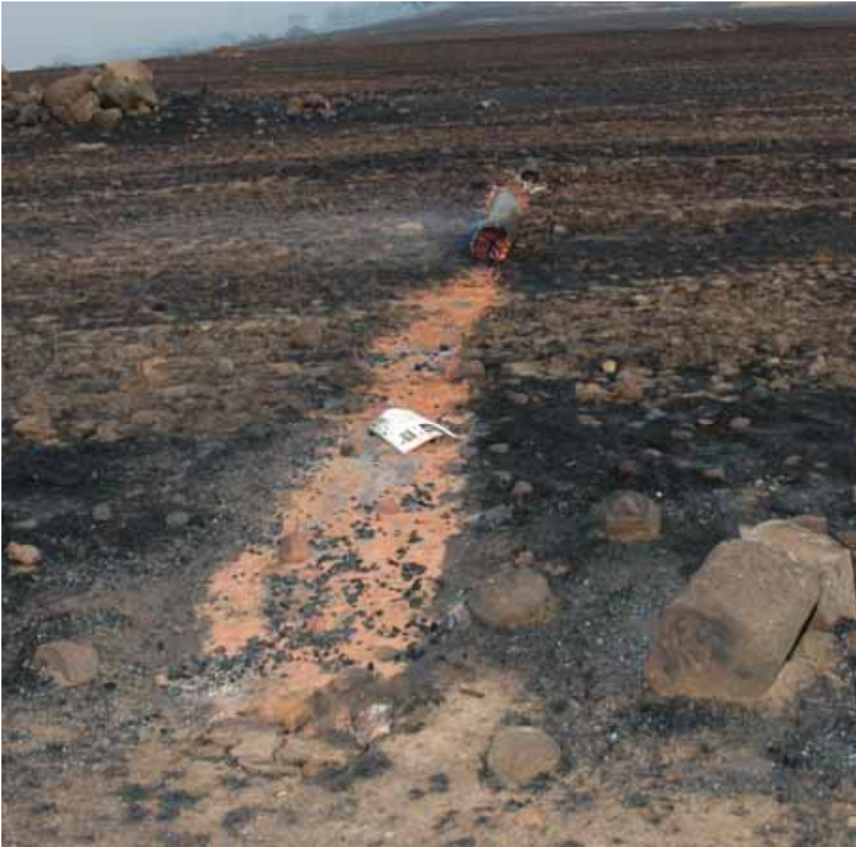
Remains of Pole T303-43. Photograph taken by FESA on 29 December 2009
