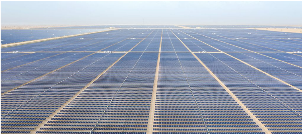
2GW Al Dhafra Solar PV project (2023), 4M modules and 20 sq km in the Abu Dhabi desert. https://www.adpv2.ae/solar-project
