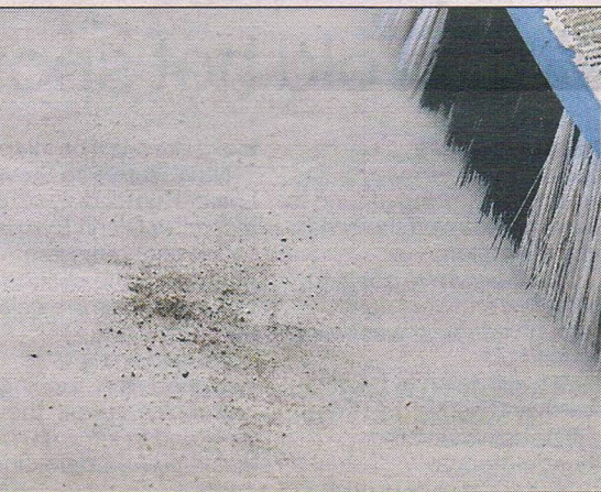
PHOTOGRAPHY: Coal dust swept up from the verandah
