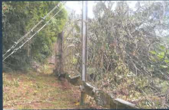
Seven rockfall fences and five berms protect the Kampong at Flying Fish Cove.
