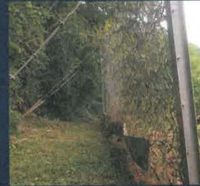
The rockfall fences are past their design life and need to be replaced.
