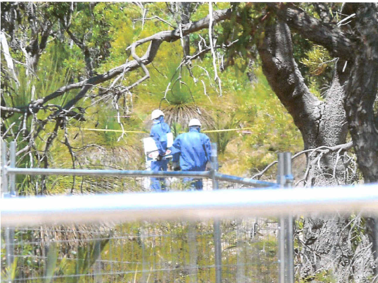
Asbestos removalists at a later stage of the Roe 8 project wearing their ppe.
