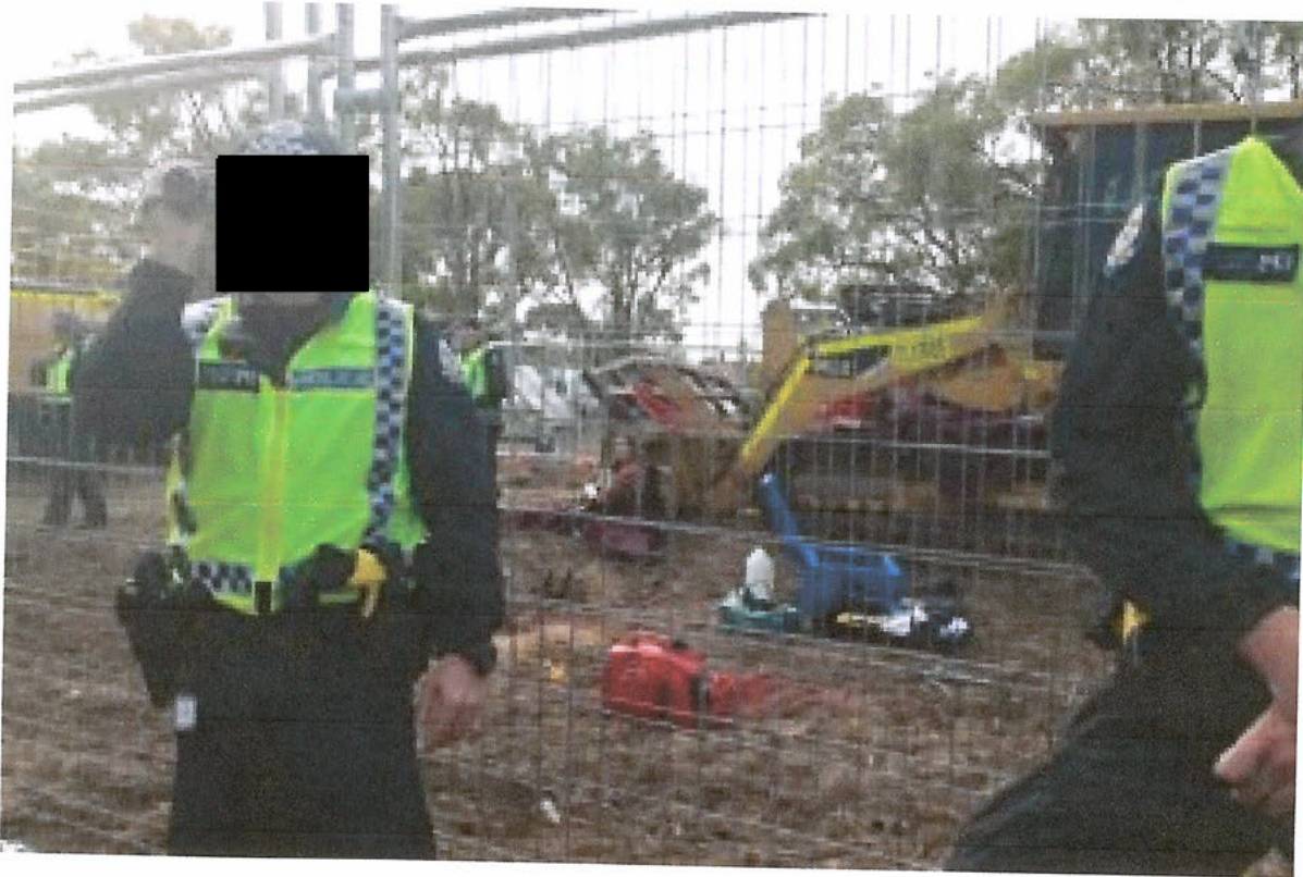
Police inside and outside the contaminated area not wearing appropriate respirators to protect them from asbestos exposure.
