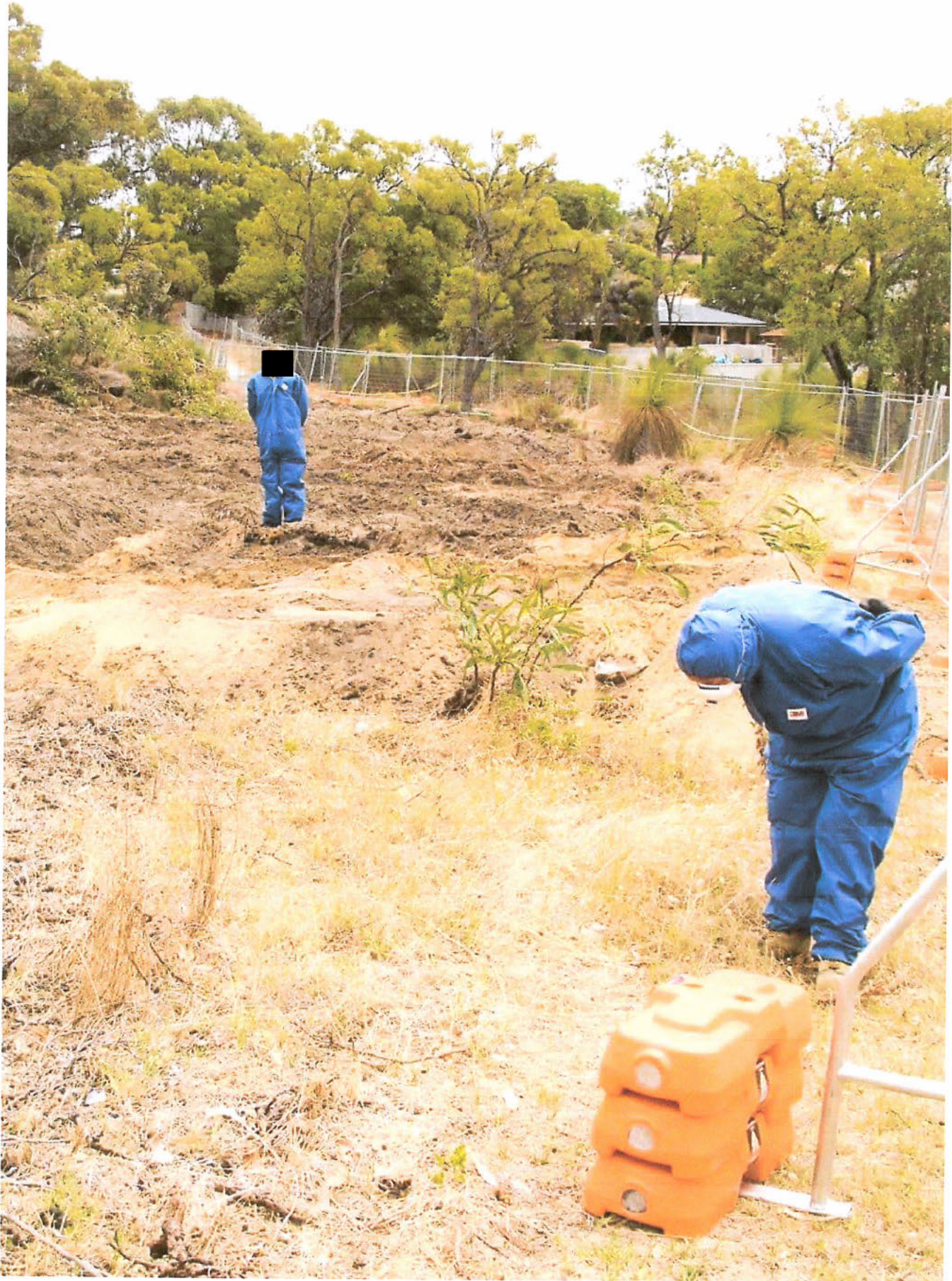
Note: One asbestos removalist is not wearing a hood as an integral part of the appropriate personal protective equipment. This is a clear breach of Section 20 of the Occupational Safety and Health Act 1984.
