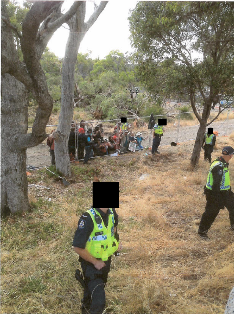
All police inside the fenced area where removal of asbestos was being conducted are not wearing ppe
