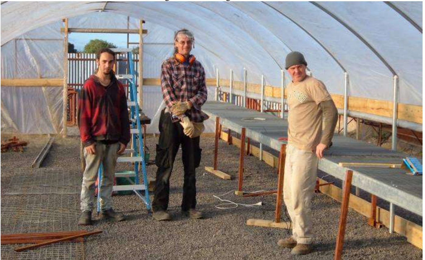
Andie and our local volunteers have been busy building nursery benches and fitting our 3 hot houses with shade cloth and automatic watering systems. They've done a fantastic job using recycled steel and lots of ingenuity!
