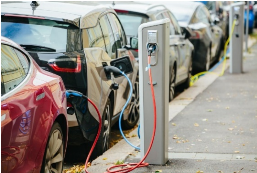
Figure 47: Static On-Street Charging Point (Source: JLLRealviews.com)
