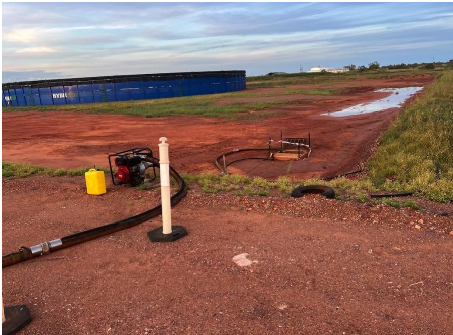
6 Hydrera Water treatment plant pumping contaminated sump water over bund wall, site entirely accessible.
