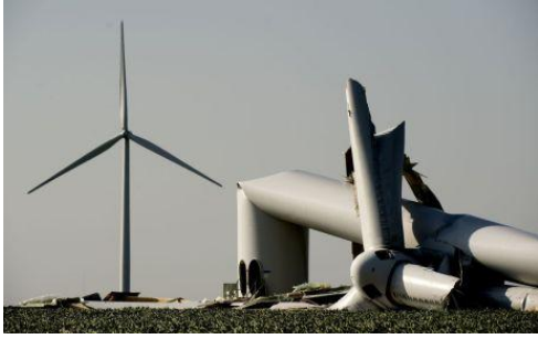
Turbines can fail catastrophically
