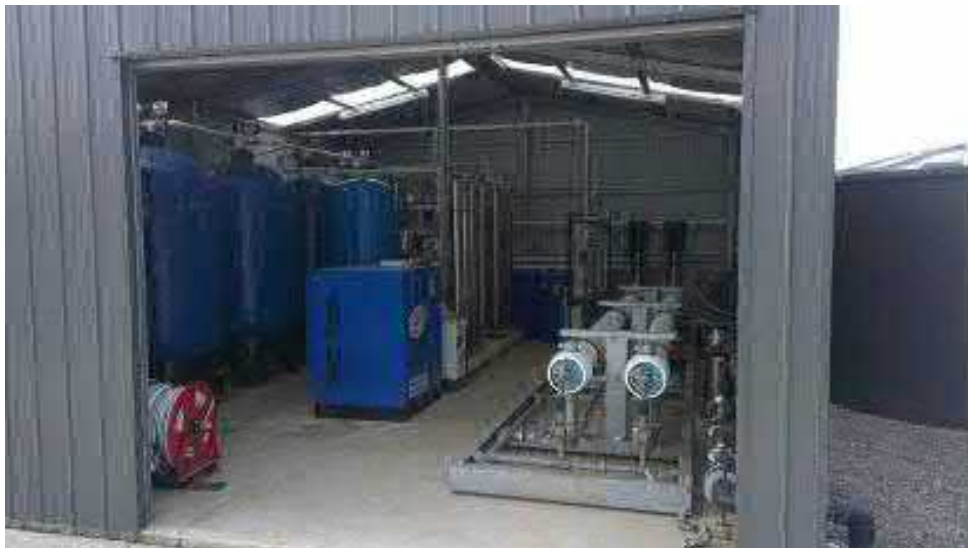
Figure 83 Desalination Plant Example (Desal Systems)
