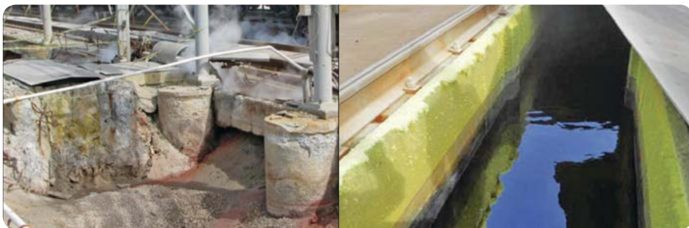
Figure 4.11: Corroded sulphur trench of Portland cement concrete at a petrochemical facility (left), and similar trench made with Ceratech's kemrock™ cement (right) after 2 years of service, showing sulphur build-up but no deterioration. 52
