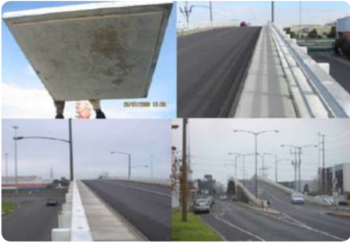
Figure 4.4: Precast footpath sections made from Zeobond's E-Crete at Salmon St Bridge, Port Melbourne
