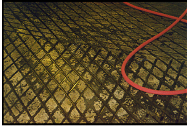
Figure 2. Diamond pattern floor that works well for pigs. The grooves are in a diamond pattern. The diamonds are 10 cm (4 in) by 13 cm (5 in). The grooves are 1 cm (0.5 in) wide by 1 cm (0.5 in) deep.
