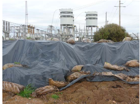
Figure 4. Evidence of the extraordinary steps taken by the community to flood-proof the electricity substation serving Kerang, Northern Victoria
