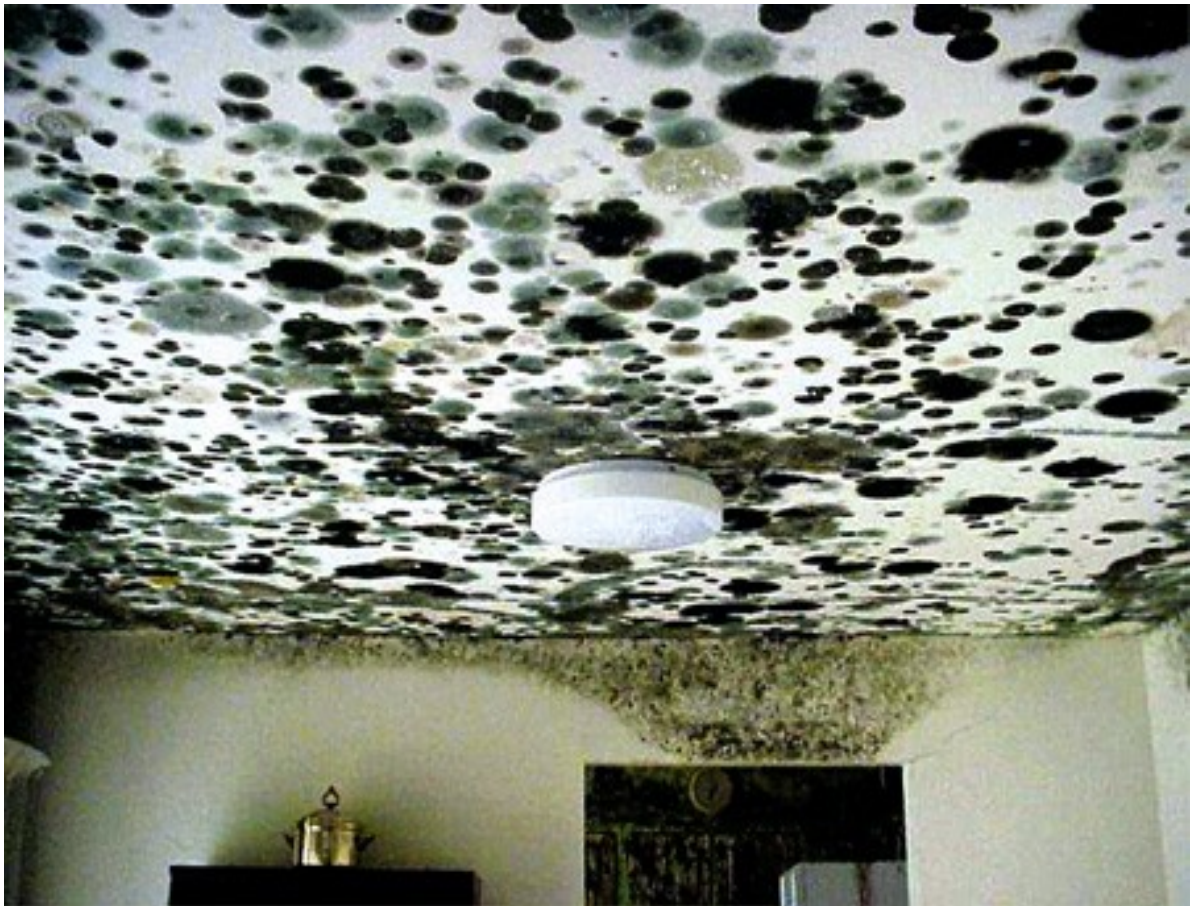
Figure 1. Mould on a ceiling due to moisture from above
