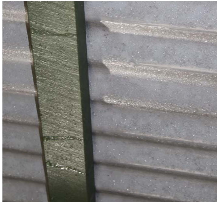
Figure 4. Condensation on the underside of a metal verandah roof
