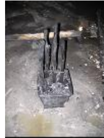
Plastic plant (post fire)
