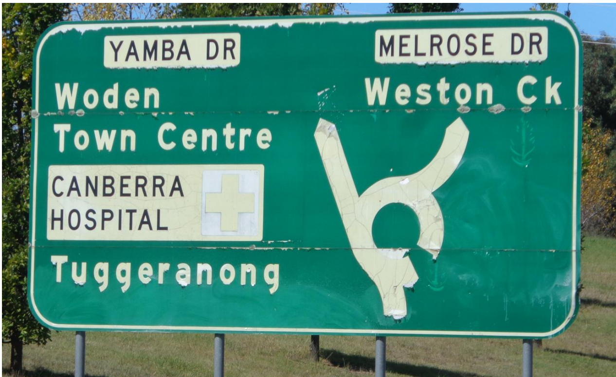
Faded, Blistering, Dilapidated Street Signs on Arterial Roads – Yarra Glen
