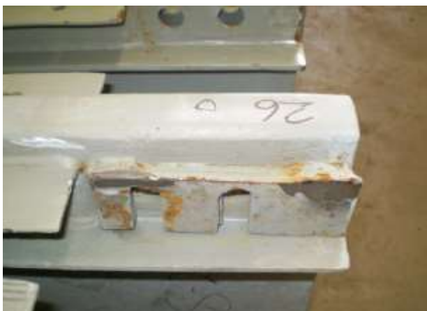
Photo 4 It is thought that the connecting chords to this beam were cut too short, requiring spacers to be inserted at each join – poor workmanship
