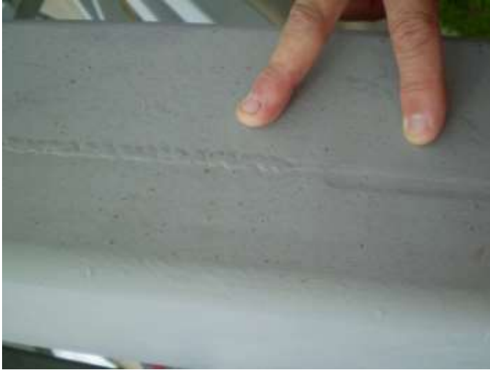
Photo 16 and 17 Poor scarfing of the weld including undercut with potential to be below the wall thickness specification.
