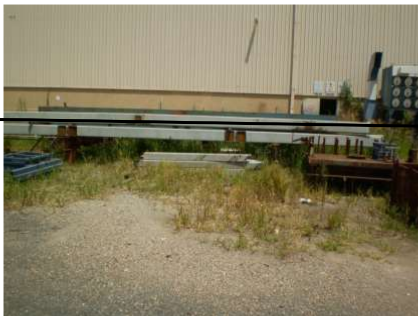
Photo 6 Bottom chords showing bending
