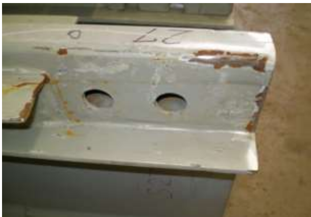
Photo 3 30mm holes were drilled to take 20 mm bolts. This is non-compliant
