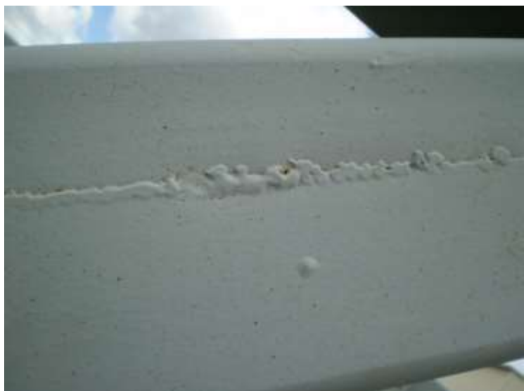
Photo 15 Very poor seam welding or rectification of an unwelded section
