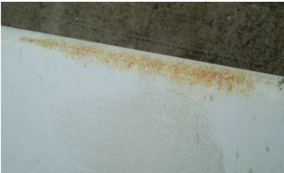
Photos 9 and 10 Poor paint finish
