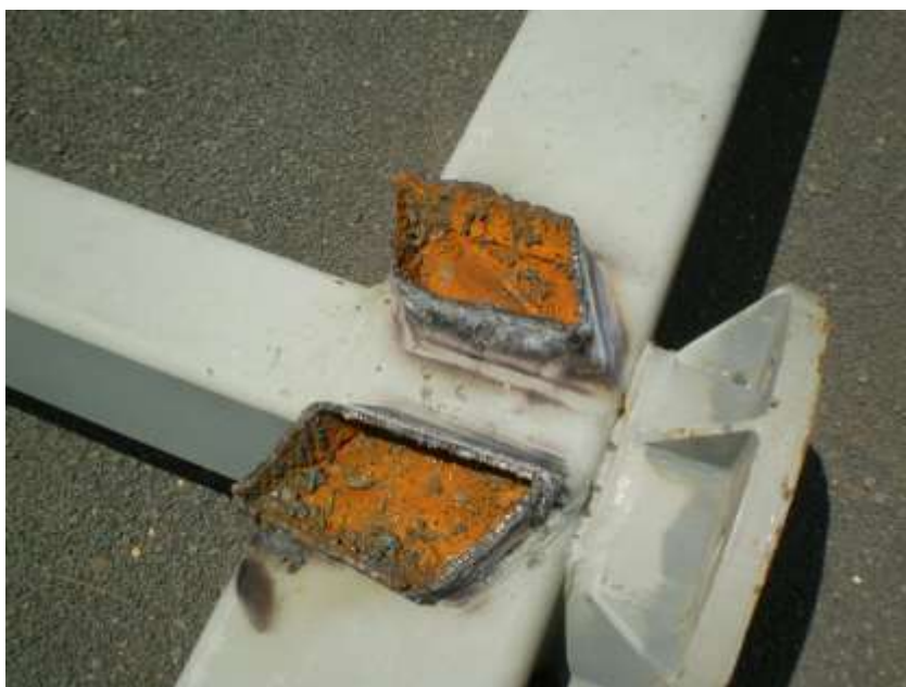
Photo 5 The diagonal chords when cut were found to be filled with water. This is extremely unusual and is thought possibly to have been deliberate to build up the weight of the structure to have a mass within overall specification.
