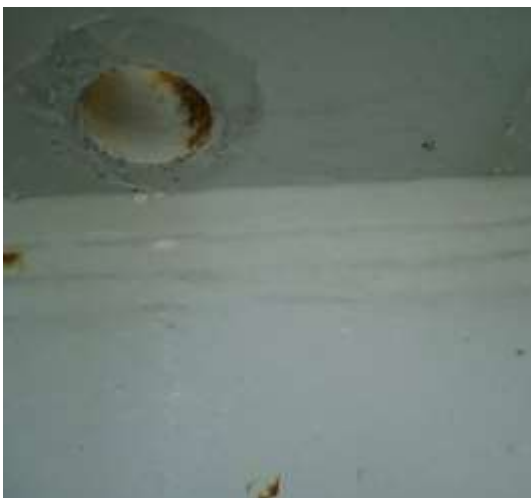
Photo 18 Fillet welds instead of full penetration butt weld
