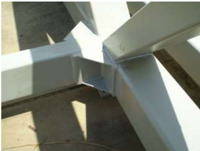
Photo 1 Showing site rectification of split join of main and cross cords of the truss
